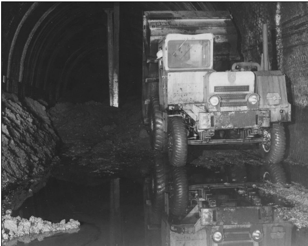
Fig. 8 Reflections in a tunnel. The SL Dumptruck completing tipping and in position to leave the tunnel.
